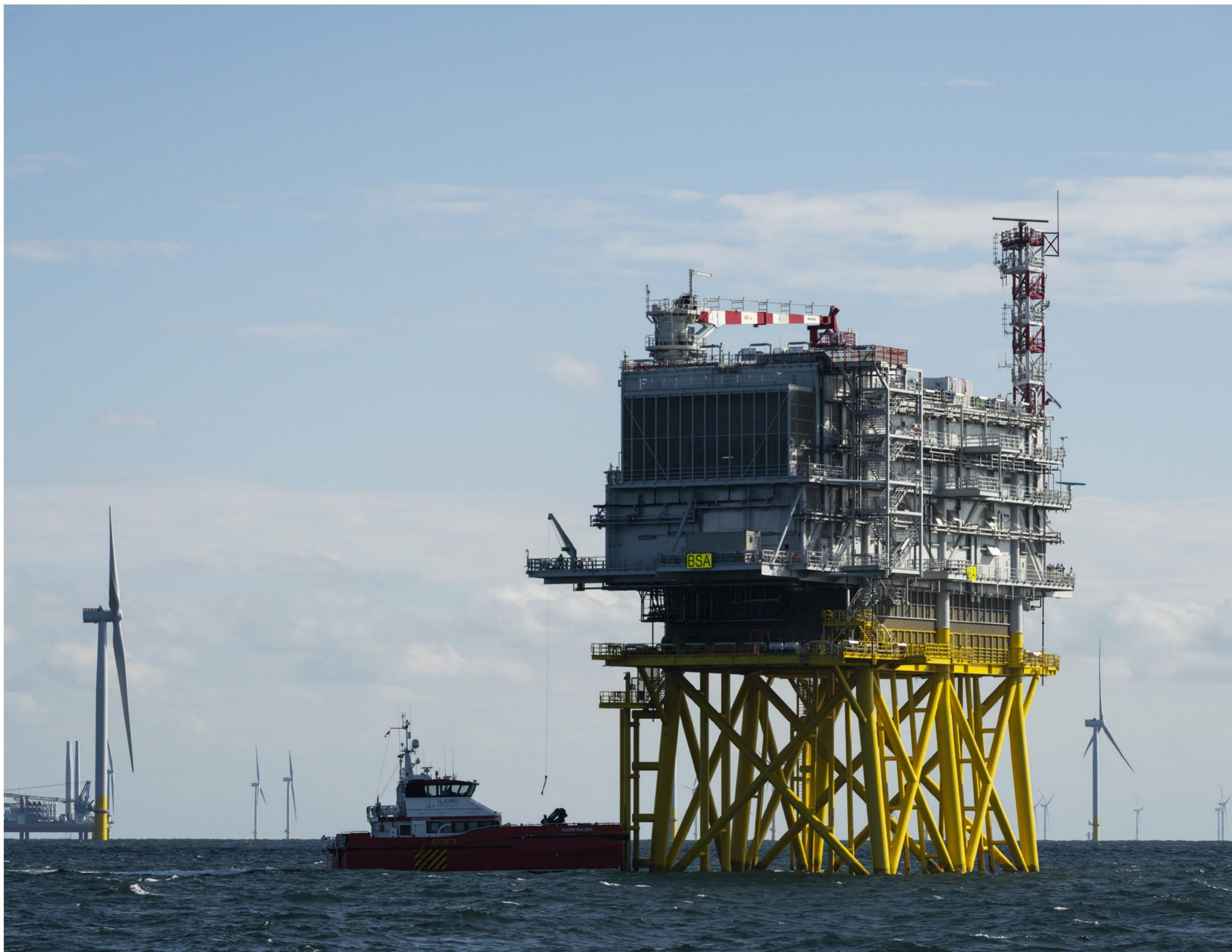
HIGH VOLTAGE OFFSHORE SUBSTATION IN BORSSELE WIND FARM, AUGUST 2020, WIND FARM OPERATOR BLAUWWIND. PICTURE SOURCE: RVO
