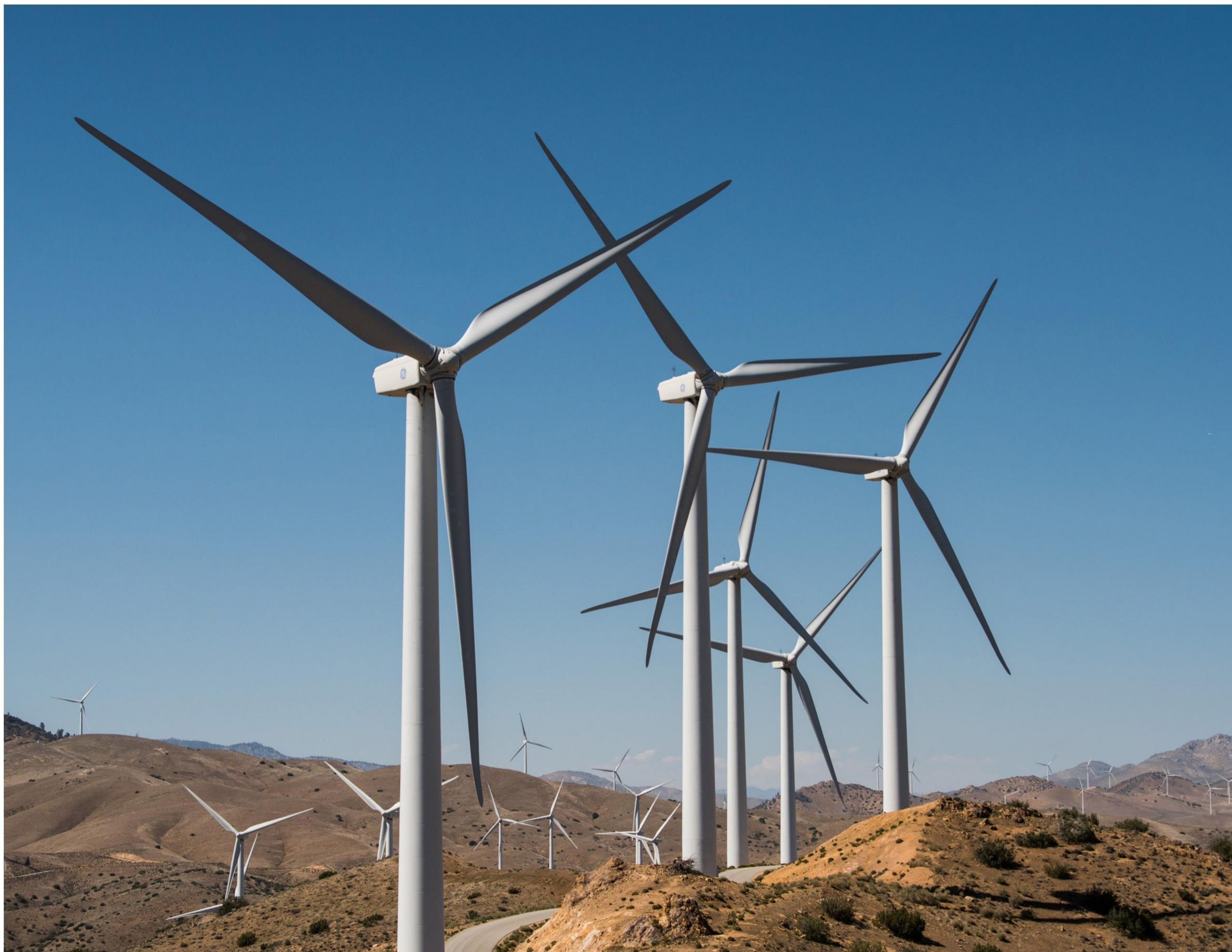
THE 8,000-ACRE LOS ANGELES DEPARTMENT OF WATER AND POWER PINE TREE WIND AND SOLAR FARM IN THE TEHACHAPI MOUNTAINS NORTH OF MOJAVE, CALIFORNIA, FEATURES 80 1.5-MEGAWATT (MW) GENERAL ELECTRIC WIND TURBINES AND IS ONE OF THE LARGEST MUNICIPALLY OWNED WIND FARMS IN THE UNITED STATES. PHOTO BY DENNIS SCHROEDER, NATIONAL RENEWABLE ENERGY LABORATORY (NREL)
