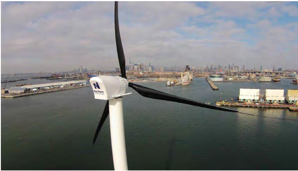
Figure 1. Medium-scale distributed wind turbine installed at an industrial complex outside of Boston Massachusetts, United States. (Source: Aegis Renewable Energy, Waitsfield, VT)
