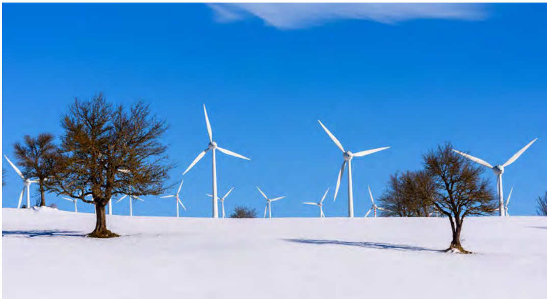
Figure 10. The E2i Energie Speciali Monteferrante Wind Farm in Italy consisting of 41 600-kW turbines
