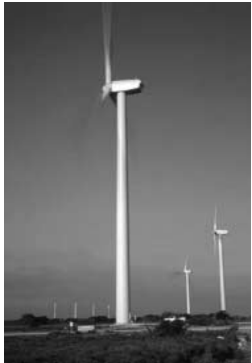
Figure 21.1 GE Wind Energy 1.5-MW turbines in 150-MW Trent Mesa wind-power plant located near Sweetwater, Texas
