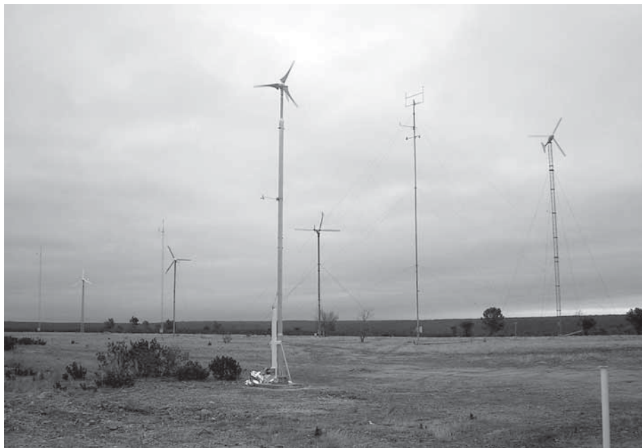
Figure 14 Small wind turbine test site.
