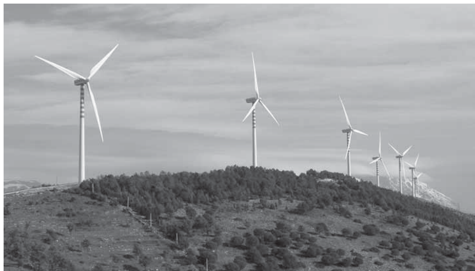
Figure 6 This 14-MW wind farm in Campania contains seven 2-MW Gamesa G83 wind turbines. Gamesa stands in the Italian market as both machine supplier and plant developer.
