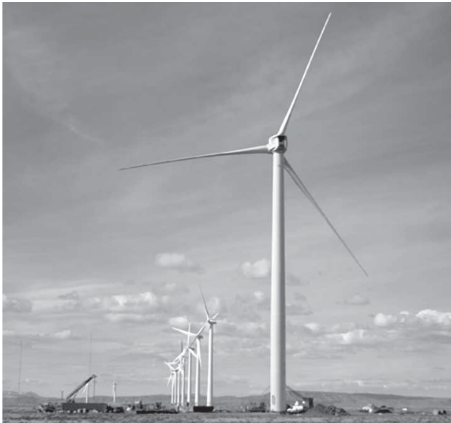
Figure 8 Clipper Windpower's 2.5-MW Liberty prototype turbine at a site in Medicine Bow, Wyoming.
