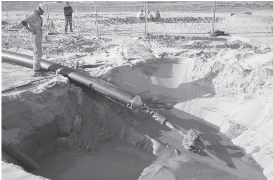
Figure 2 Tubing for cables Offshore Wind farm Egmond aan Zee. Photo courtesy NoordzeeWind.
