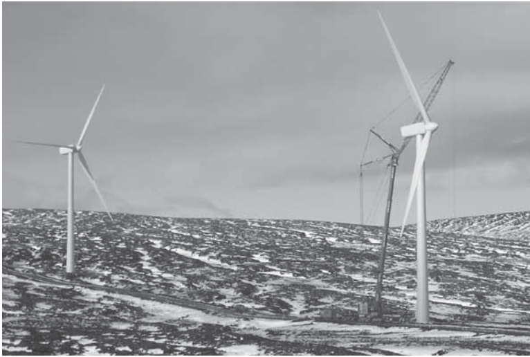
Figure 1 Braes O' Doune Wind Farm being completed in early 2007, Dunblane, Scotland (photo courtesy of Airtricity Developments UK Ltd ).
