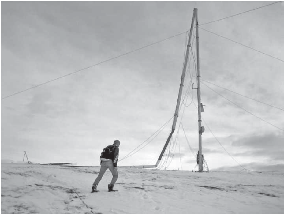
Figure 6 Measuring tower overturned due to heavy icing and high wind gusts at Schwyberg, 12 November 2007.
