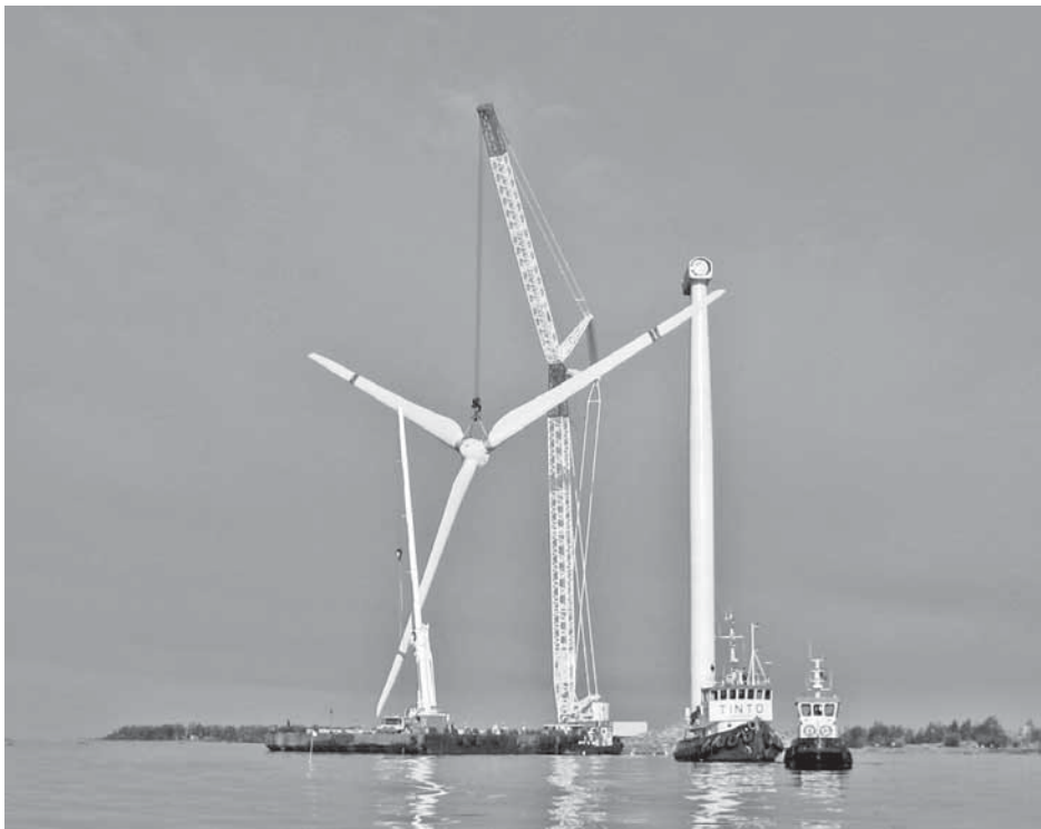
Figure 4 Erecting semi-offshore wind turbine in Kemi, where ten 3-MW turbines are to be built in 2007 and 2008. (Photo: WinwinD).
