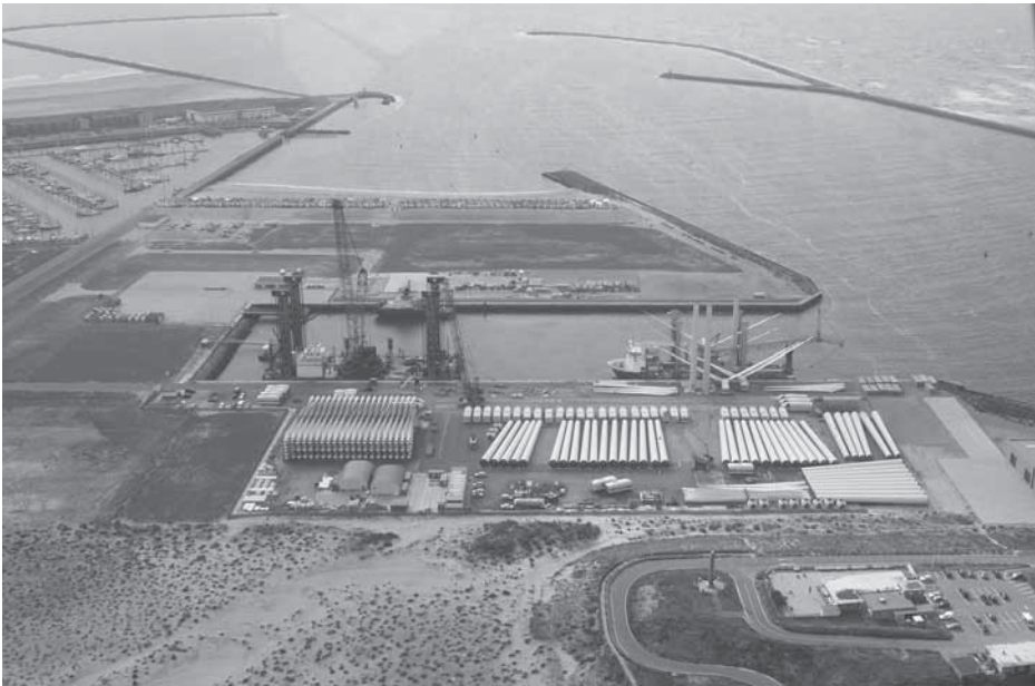
Figure 4 Q7 construction yard at IJmuiden Harbour on 27 July 2007, towers, blades, and nacelles. Photo: Jaap 't Hooft, SenterNovem.
