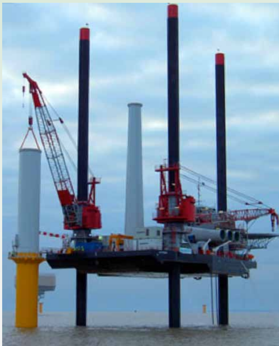
Figure 1 Gunfleet Sands Offshore Wind farm under construction (Image courtesy of Seatrax Inc and Semco Inc.)
