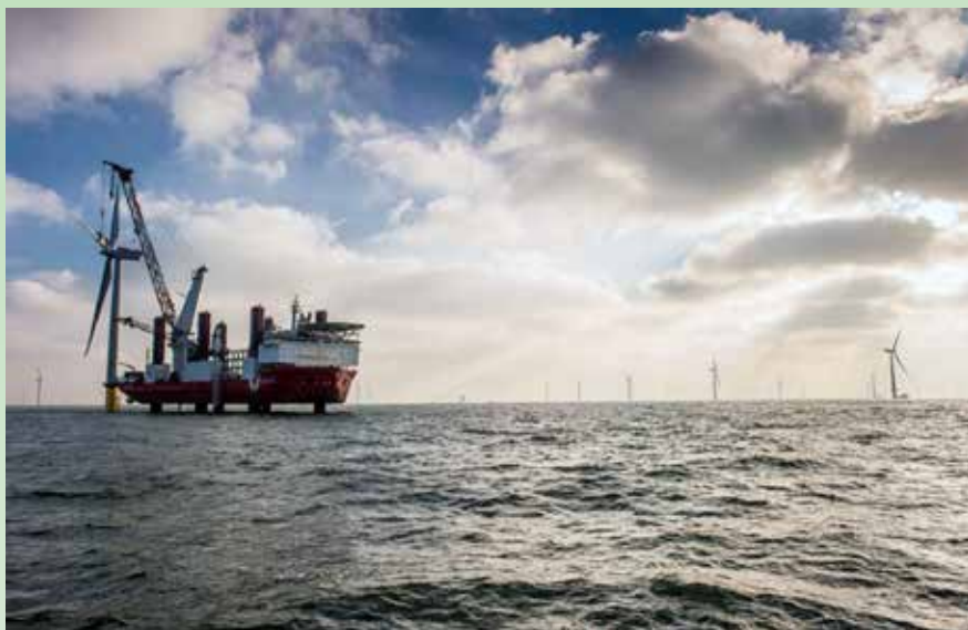
Figure 2. Installation of final turbine in first 630-MW phase of the London Array Offshore Wind Farm. Courtesy: London Array
