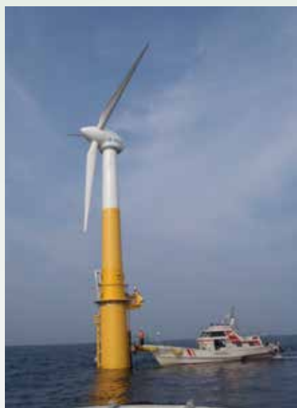
Figure 3. A small-scale floating offshore wind turbine (SUBARU 22/100 100-kW) installed 1 km offshore in Nagasaki Prefecture in the MOE Floating Offshore Wind Turbine Project
