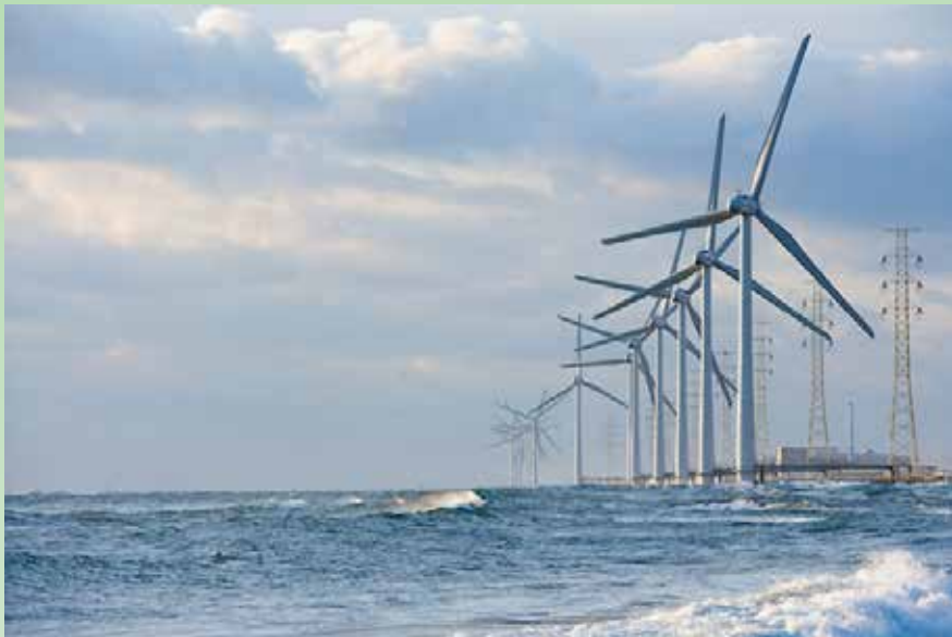
Figure 2. Wind Power Kamisu No. 2 offshore wind power plant in Ibaraki prefecture (Source: Komatsuzaki Urban Development Corporation)
