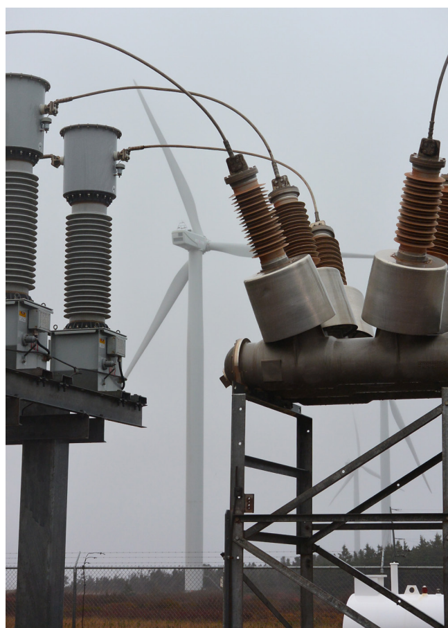
Figure 11. High-voltage direct current transmission (Photo credit: R. Hinrichs)
