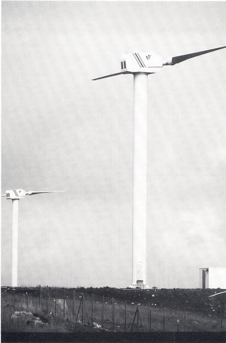
Figure 2.4.2 Partial view of the wind farm set up by WEST near Bisaccia in the Campania region
