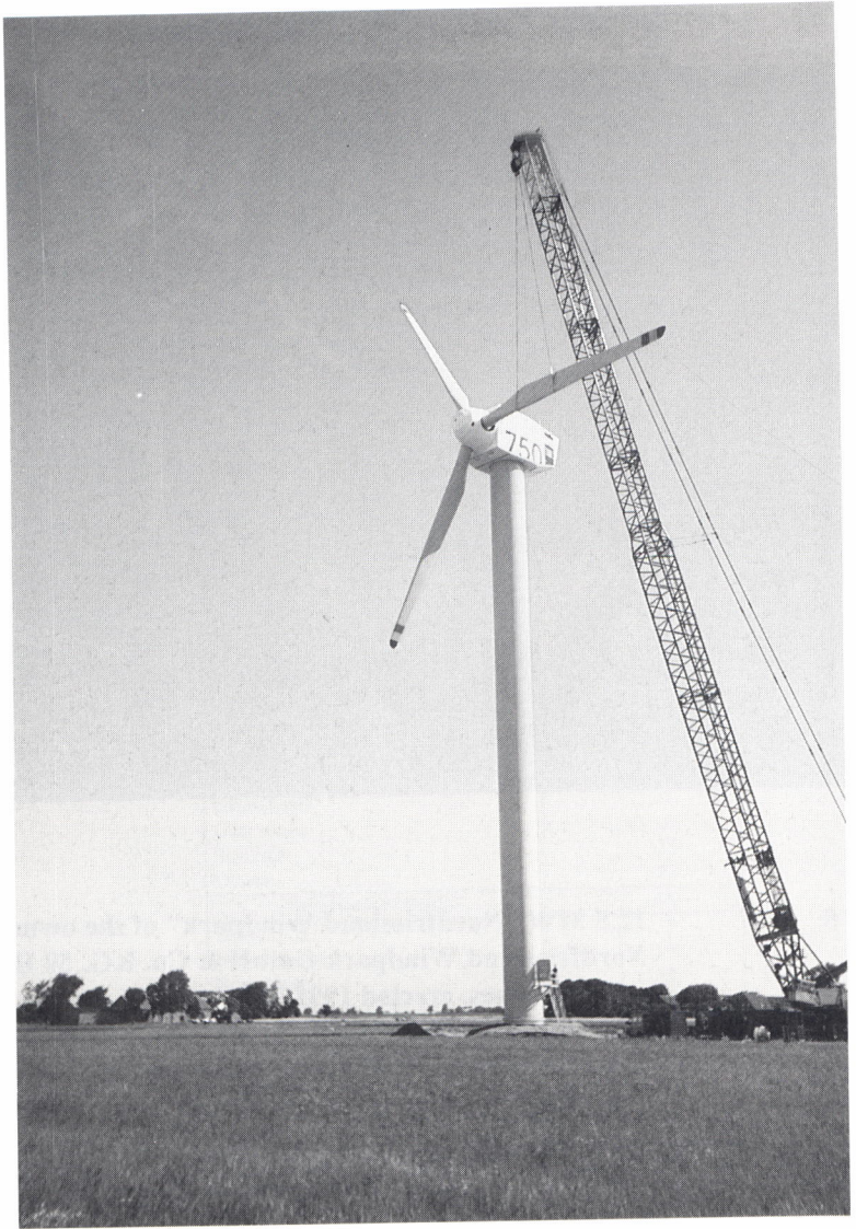
Fig. 6 HSW 750 at the Kaiser-Wilhelm-Koog test facility. Rotor diameter 40 m, hub height 45 m. Mean annual wind speed at hub height 7,0 - 7,5 m/s.
