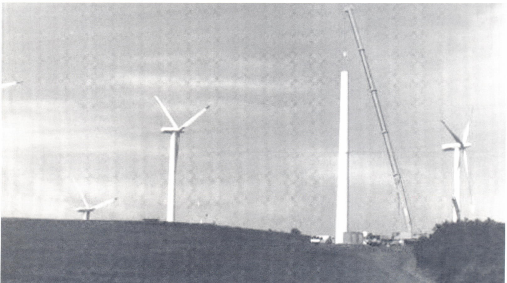
Figure 14.4 Machine erection at the wind farm built by Filippo Sanseverino near Castelfranco in Miscano (Campania) with 50 units totaling 30 MW
