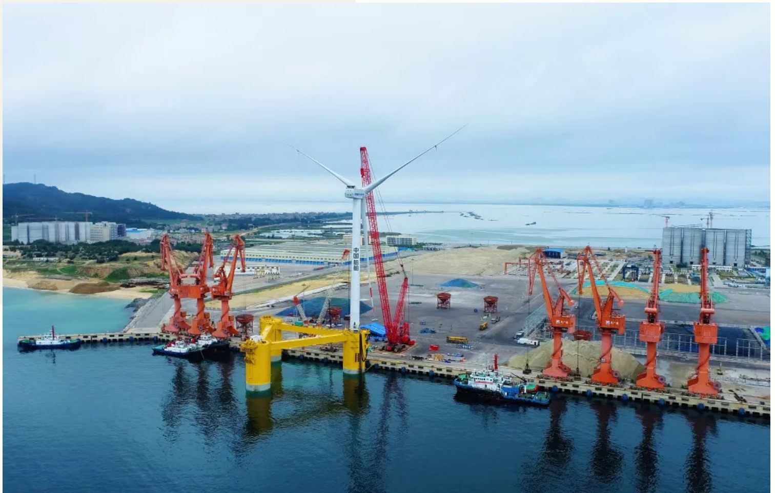
“Fuyao” wind turbine is installed on the floating platform at the Port of Maoming. Photo: China Haizhaung
