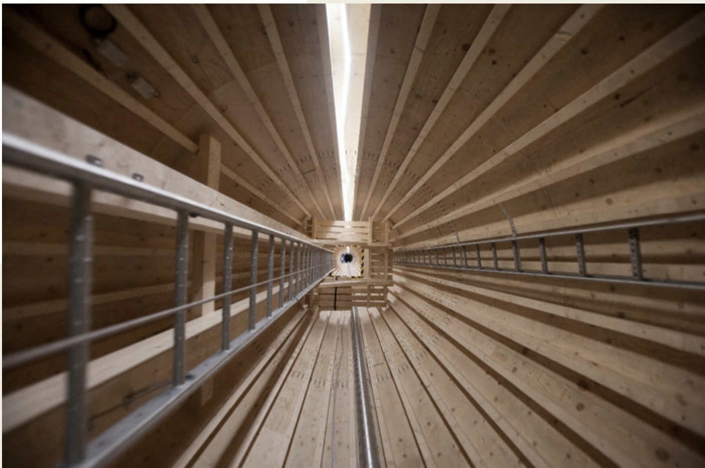
Inside view of the 30 m wooden tower from Modvion on Björkö (Gothenburg) (Source: Modvion).
