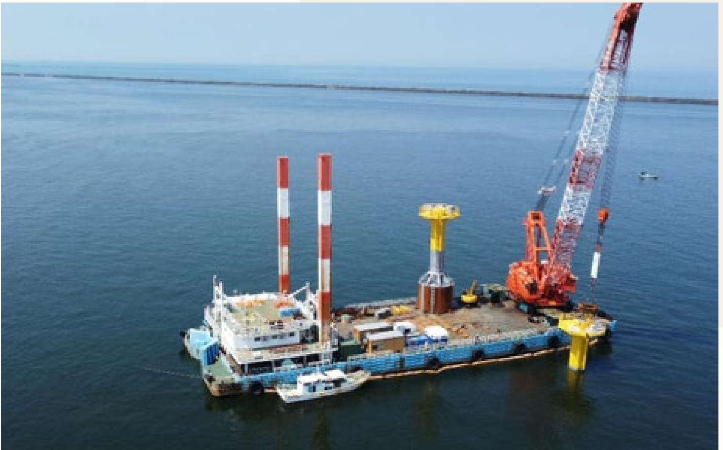
Figure 3: Demonstration of base construction technology for suction buckets in actual sea area.
