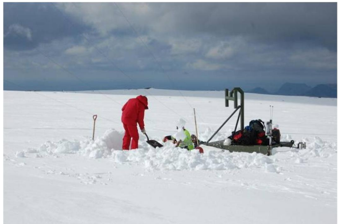
Figure 4-3 Accessing power system in a remote location. The whole 2.5-meter high container apart from the air inlet to the engine has been buried. Photo credit: Lars Tallhaug, Norway
