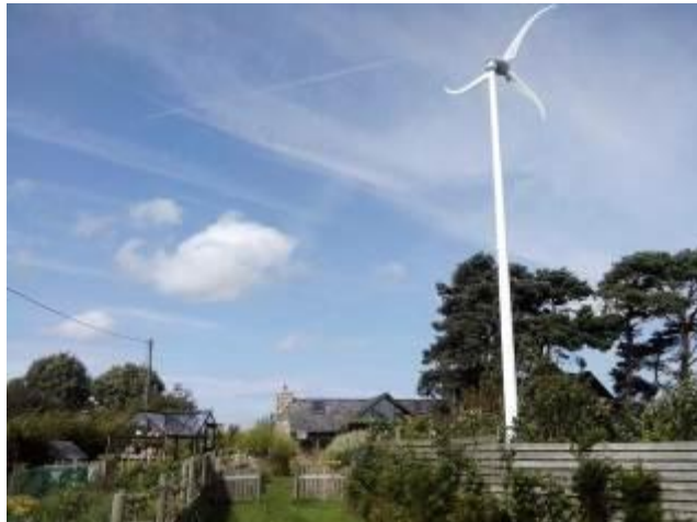
Figure B.10. Skystream wind turbine at Site B
