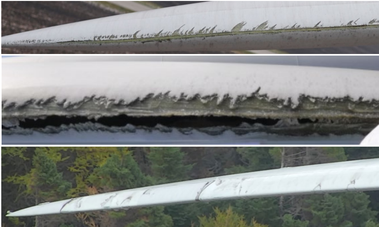
Figure 2-1 – Examples of wind turbine blade erosion damage (top - progression of leading edge erosion, middle – untreated leading edge erosion resulting in open cavity, bottom – damage to leading edge protection tape).
