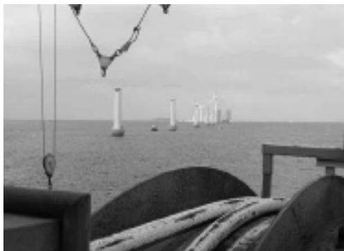
Figure 10.5 The Middelgrunden wind farm under construction. Photo by Jens H. Larsen and Mads Eskesen. Published with the permission of Københavns Miljø og Energikontor.
