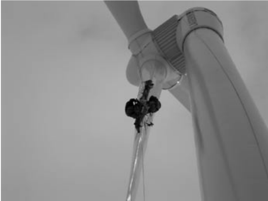
Figure 19.3 Repairing blades of the 800-kW wind turbine on Mount Gütsch, 2,300 m above sea level in Andermatt, Switzerland
