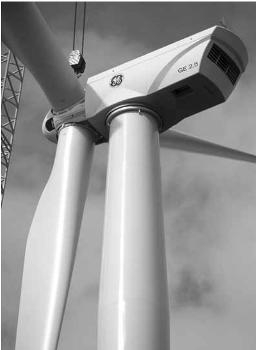
Figure 4 Erection of the GE Wind 2.5-MW turbine at the ECN test site. Photo courtesy of General Electric Wind.
