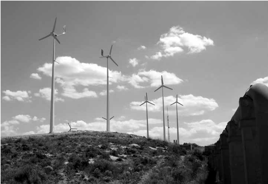
Figure 8 Wind farm with small wind turbines (5kW grid connected).
