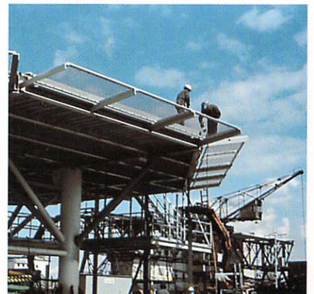
Helideck to the "Danfield platform E", The North Sea.
