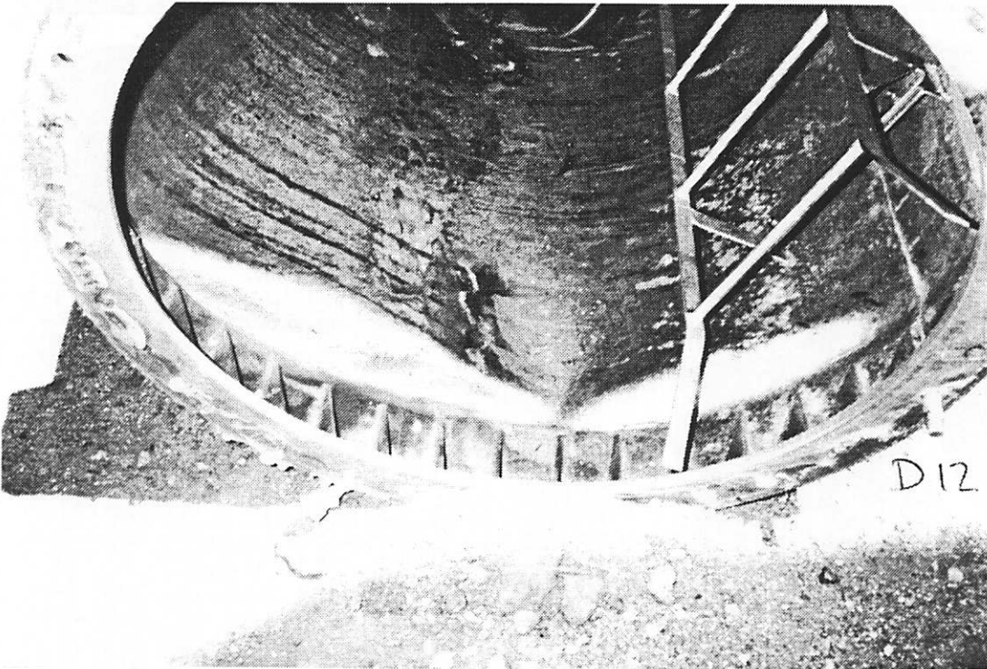
4 Buckling zone of wind turbines D12.
