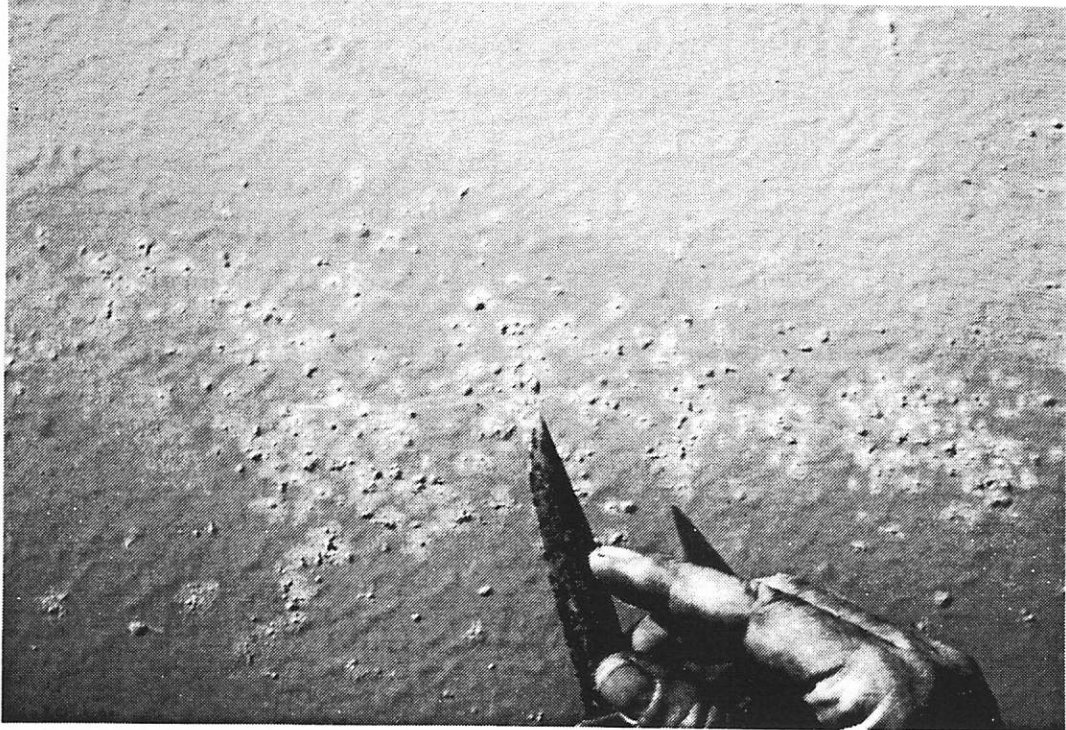
10 Oxide spots on the tower surface/Somalia.
