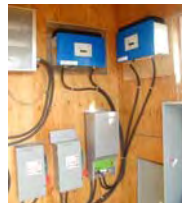
Two 1800-Watt Windy Boy inverters connected in parallel in single-phase 120/240 V.
