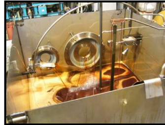
Lube System Flow Rate
