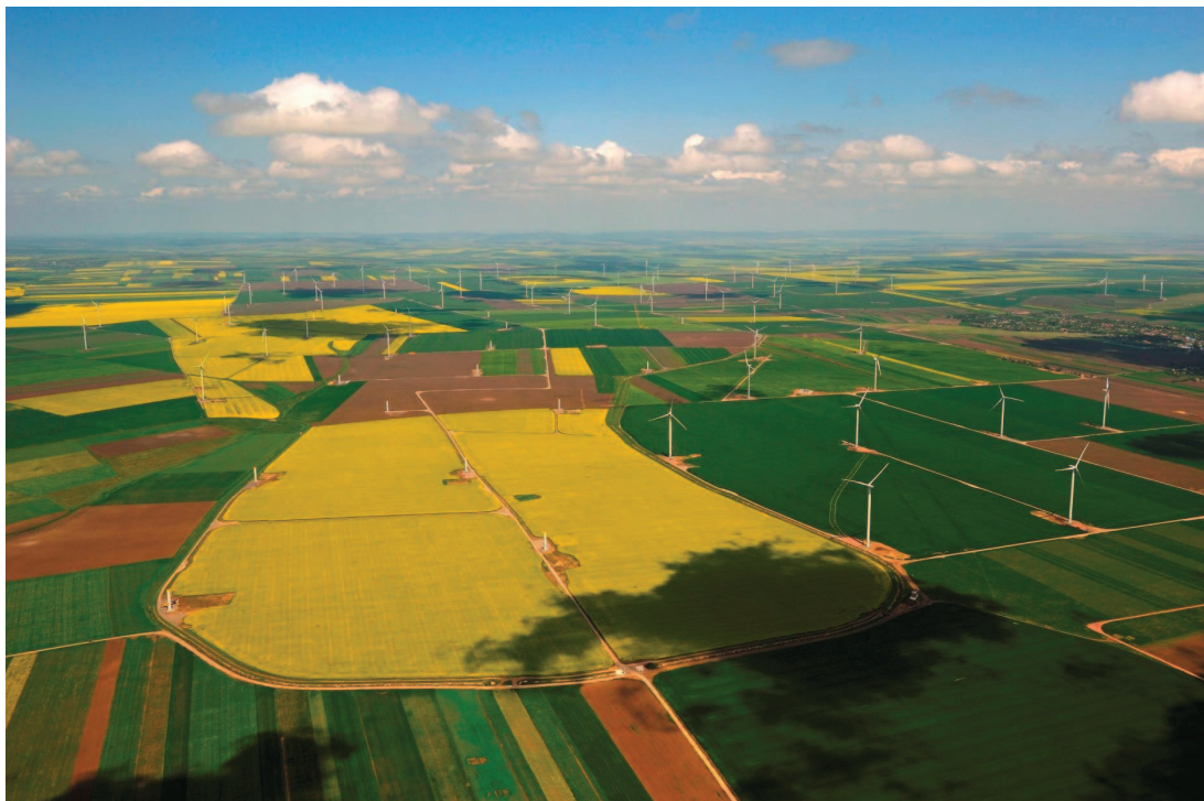
Fantanele-Cogealac, Romania: 240 GE 2.5 MW wind turbines, 600 MW farm power. Installation was completed in November 2012
