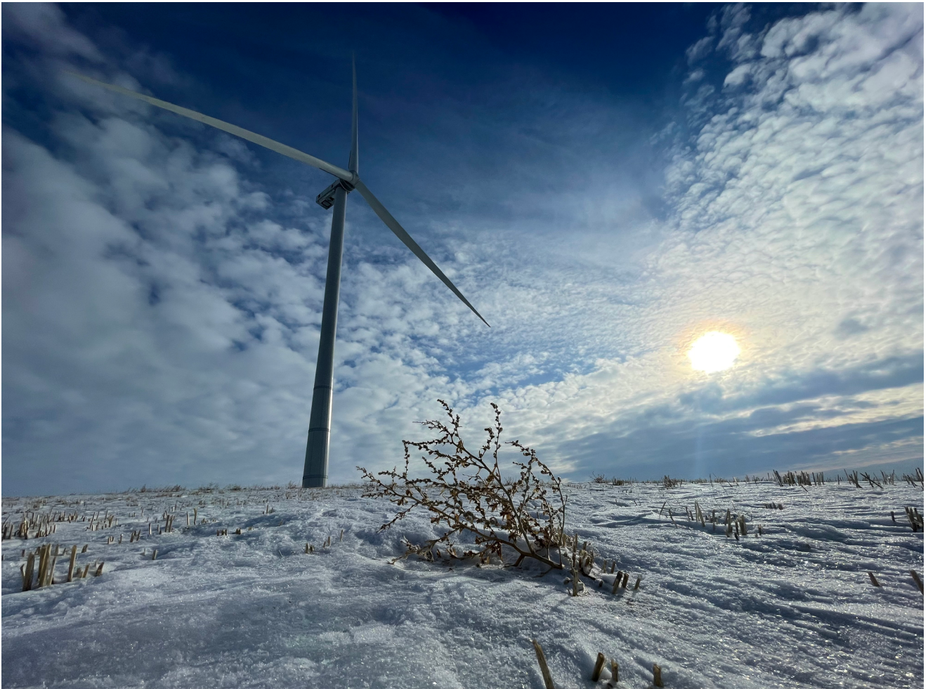
Photo 1: The three-phase 409 MW Jenner Wind Project, under construction in Alberta, features 55 Enercon E-160 EP5 E3 turbines. Credit: ENERCON Canada Inc.
