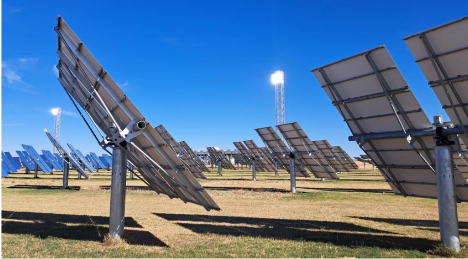
Heliostat mirrors in operation
