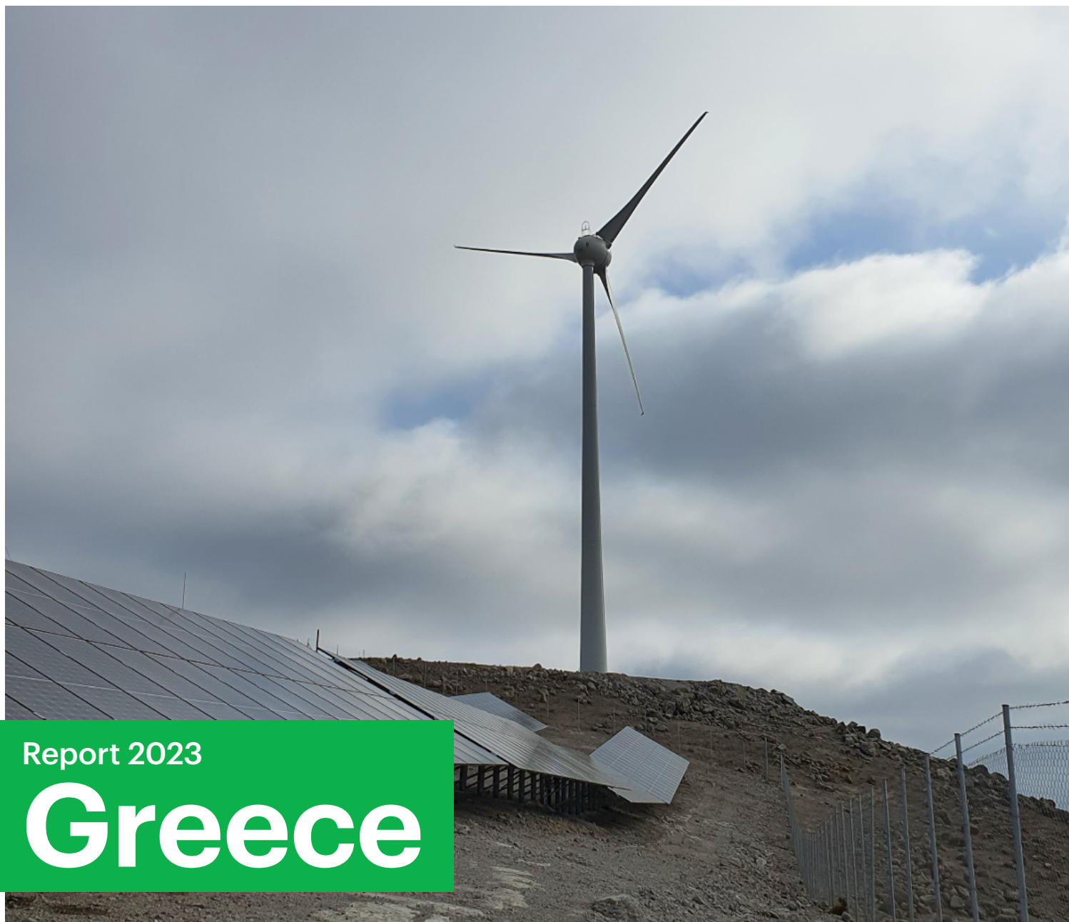
Wind turbine and PV panels at the Hybrid complex in Agios Efstratios island, North Aegean, Greece. Photo: CRES.
