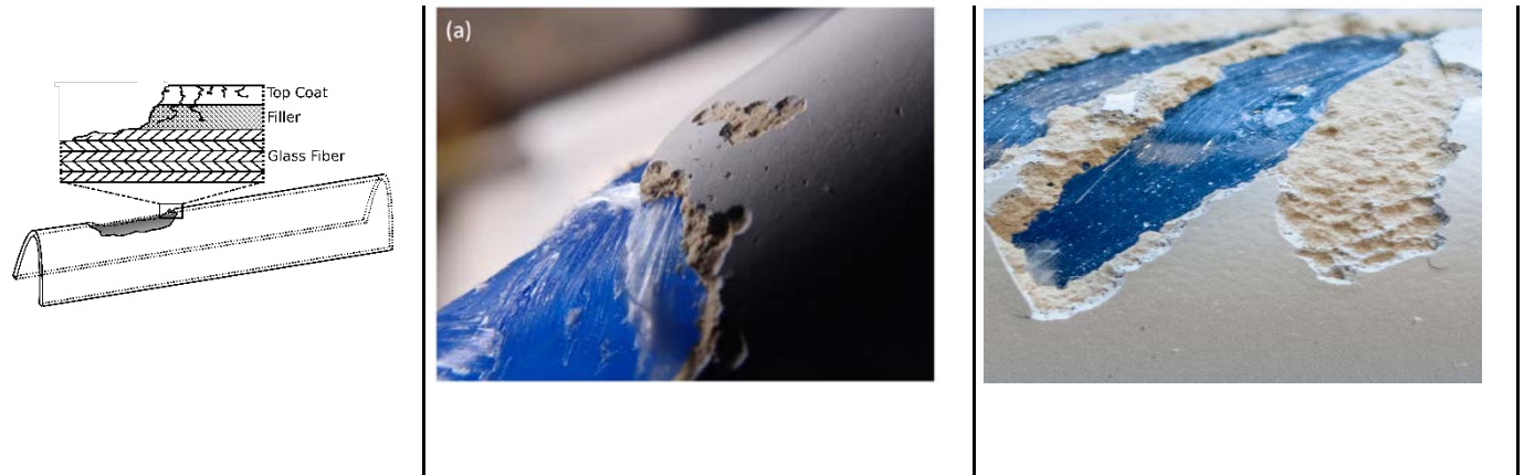
Figure 8: Breakthrough to substrate – cohesive failure.
