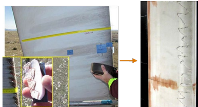
Figure 10. Field measurements and wind tunnel test of Cat 4 erosion (Ehrmann & White, 2015) (Maniaci, et al., 2016)
